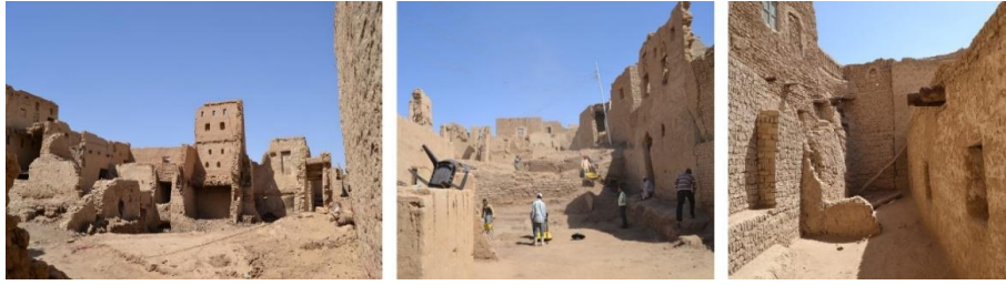
Fig. 20. Project of the restoration of the village using the same building materials and mud brick with popular participation.
