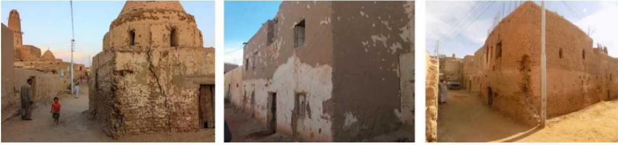
Fig. 17. Homes that are cracked and have a lot of problems in Al-Qasr.
