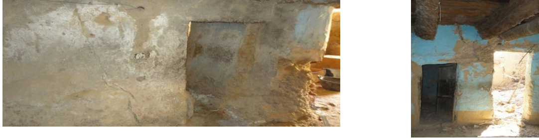
Fig. 3. Structure system in Siwa Oasis Kerchief bearing walls and palm trunks called (Fatimi).
